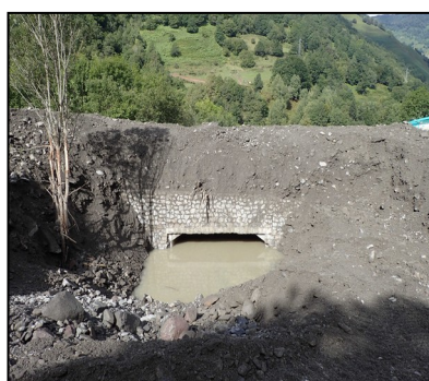
Figure 30: OH hydraulique comblé
